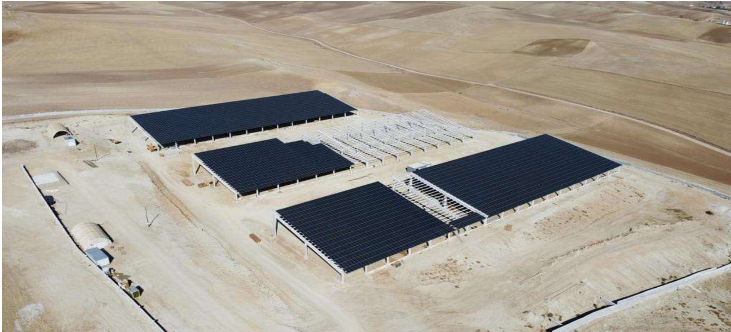
2MW GES 2020 AKSARAY/TURKEY
